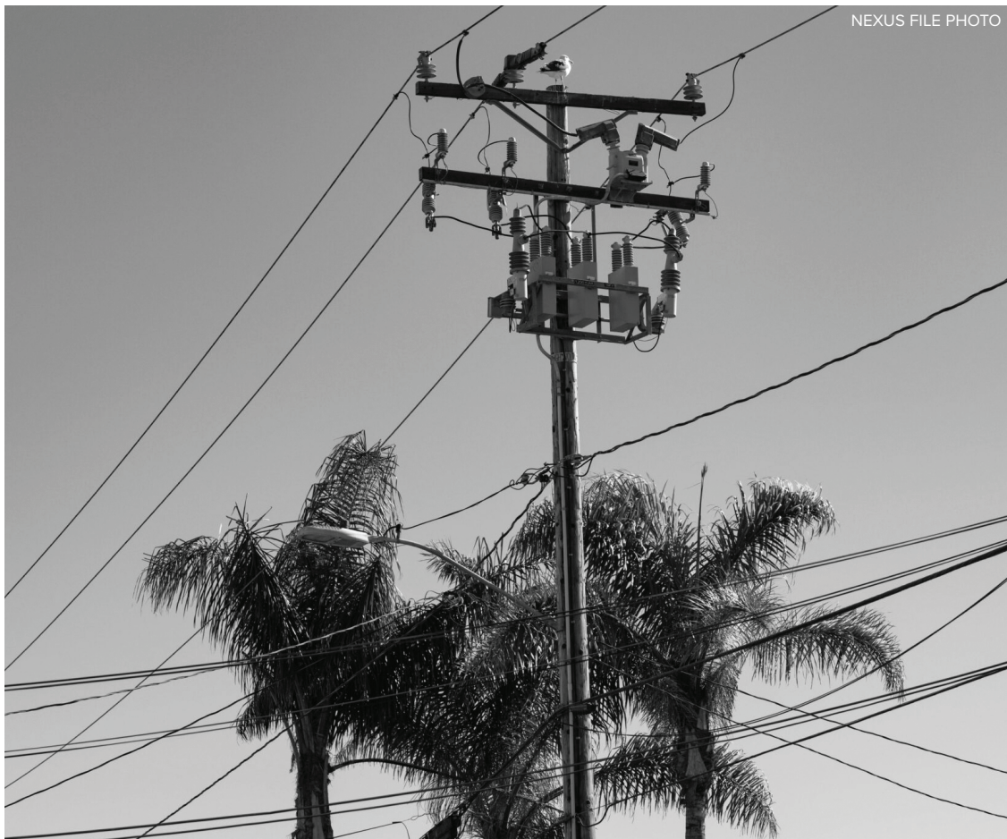
The microgrid will be “clustered around” People’s Park with the main power lines affected running down Embarcadero and Trigo Road.
